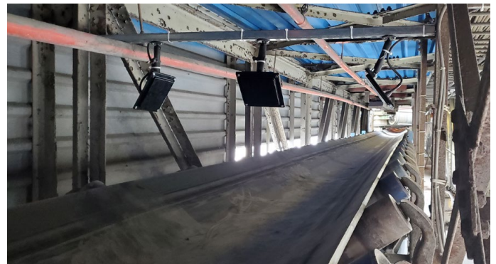
TopVu OTS checkpoint at Boliden Tara in Ireland.
