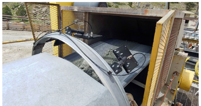
Upper West and East side ore belt installation (muck from above surface elevation hauled by train).
