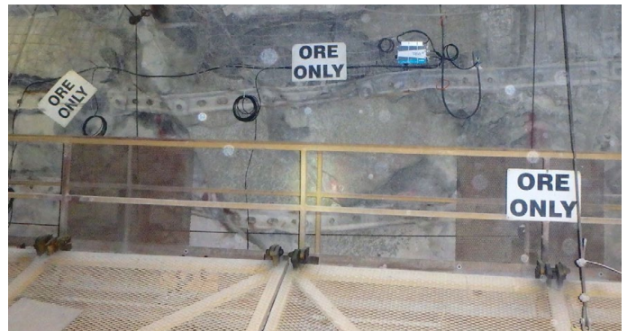
Example of underground rail dump installation.
